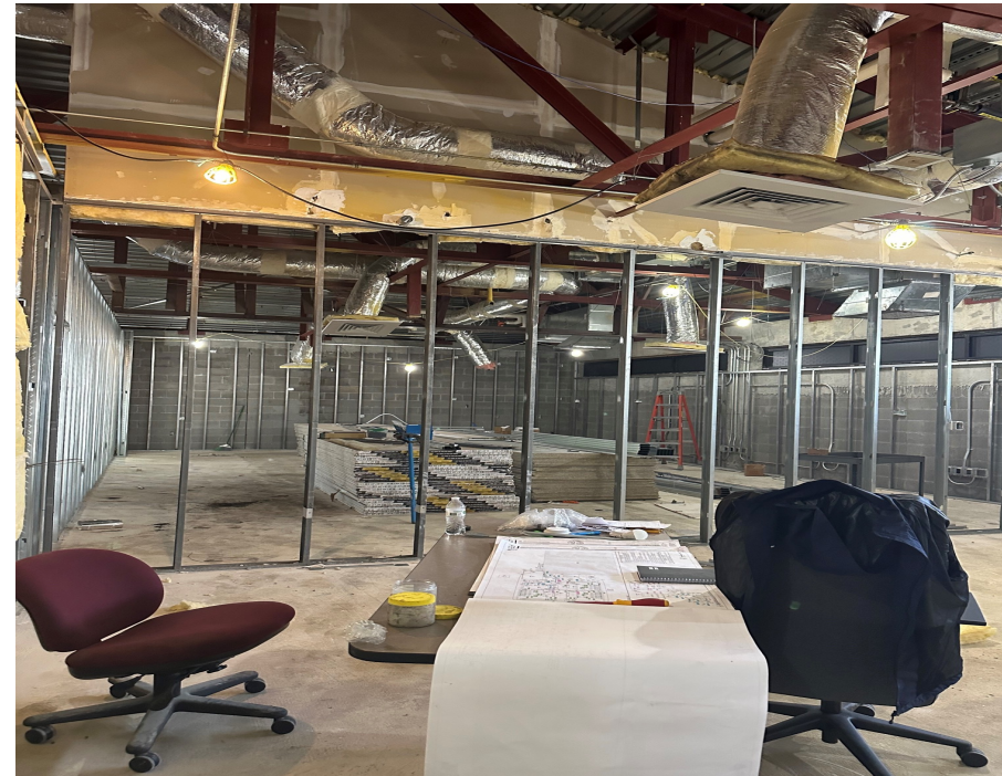
Building 2901 - AHUs and Ducts – In Progress
