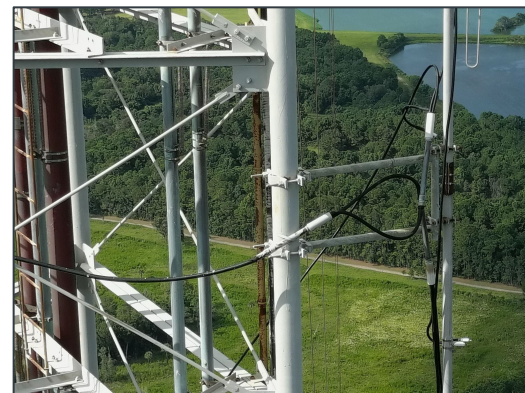
UAS visual of needed repairs for NOAA Weather Radio tower
